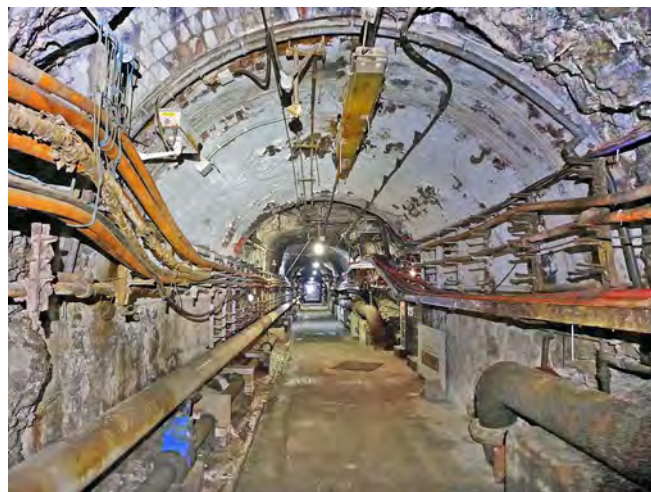
Admiralty Tunnel: lined and rock-cut sections, with the accretion of many generations of pipework and cabling
